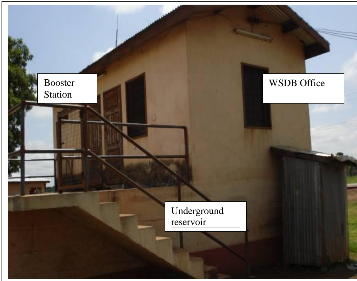
Picture 1: Underground Reservoir, WSDB Office and Booster Station
